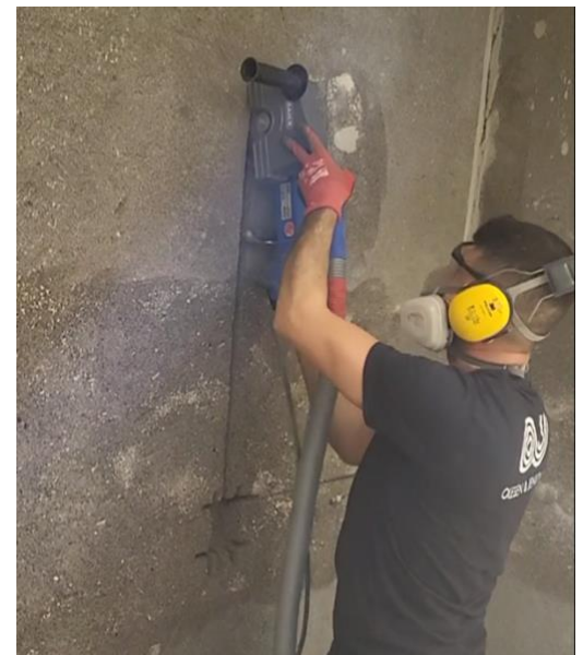
Automating channel cutting for wiring can help improve electricians' working environment. Depending on the complexity, the task can be automated to varying degrees. Photo: Bjarke Reggelsen, HowToRobot.
