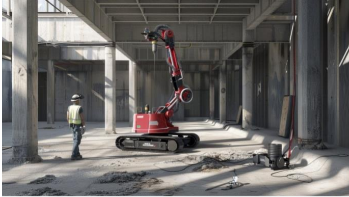
Mobile drilling robots can aid electricians but may require some adjustments at construction sites. Image: AI generated
